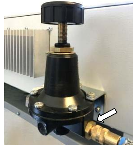
Figure 12: Compressed air connection on the pressure regulator
